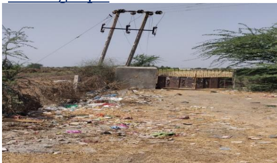
Fig. no.6.1a current situation of cleanness
