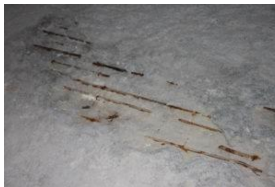
Fig. 5.1.2a when the signs of damage became visible of corrosion
